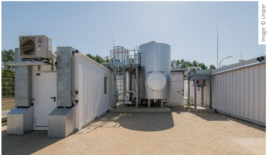
Figure 1: The methanation demo plant in Falkenhagen, Germany, was the first one of STORE&GO's three demo sites that went operational
